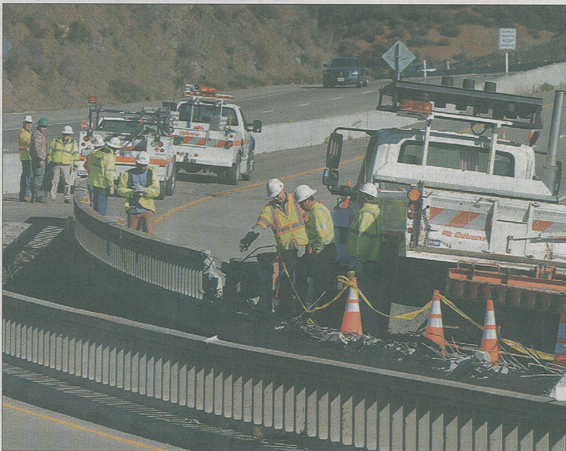
Caltrans workers inspect the bridge and plan their course of action following the crash.
