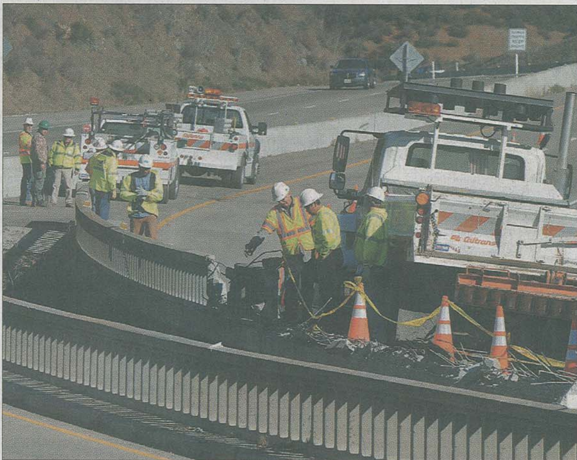
Caltrans workers inspect the bridge and plan their course of action following the crash.
